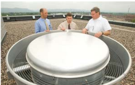
Retrocommissioning efforts on several hundred exhaust fans of various uses and sizes have been made as fans run only when needed and reduce energy consumption.
