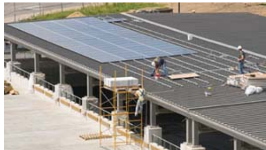
Solar panels installed on the roof of Gundersen Lutheran's new underground parking ramp produce electricity to help power the structure.
